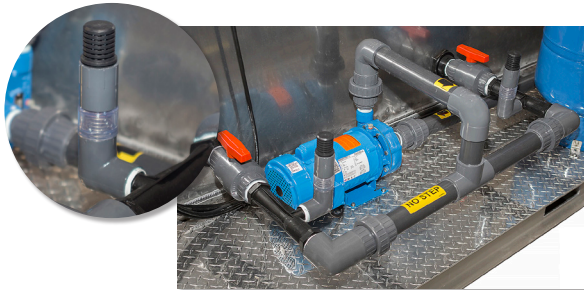
Mazzei® venturi air injection system, 55-0126, sustains beneficial aerobic microbes while preventing bacteria from turning odorous and anaerobic
